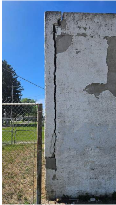
Figure B10 - Item S3 – Shop wall vertical crack in CMU wall.
