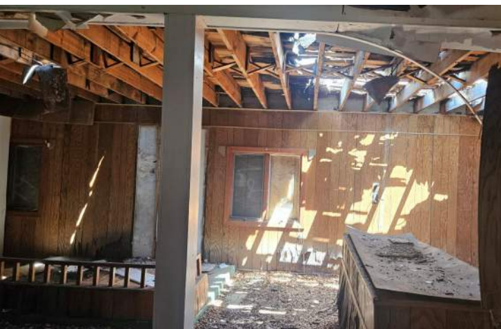
Figure A19 - Item S4 – Typical Roof Framing over Office Wing – partial roof decking collapse.
