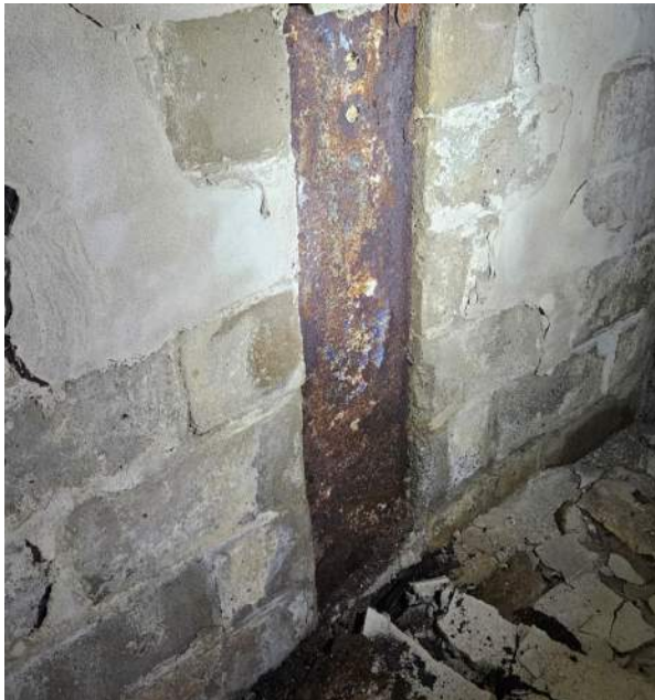
Figure A9 - Item S1, S2 – Corroded steel column supporting floor beam above in Office Wing.
