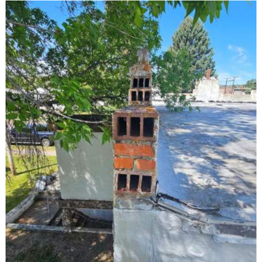
Figure A16 - Item S4 – Office Wing Terra-Cotta parapet wall – unreinforced and ungrouted.
