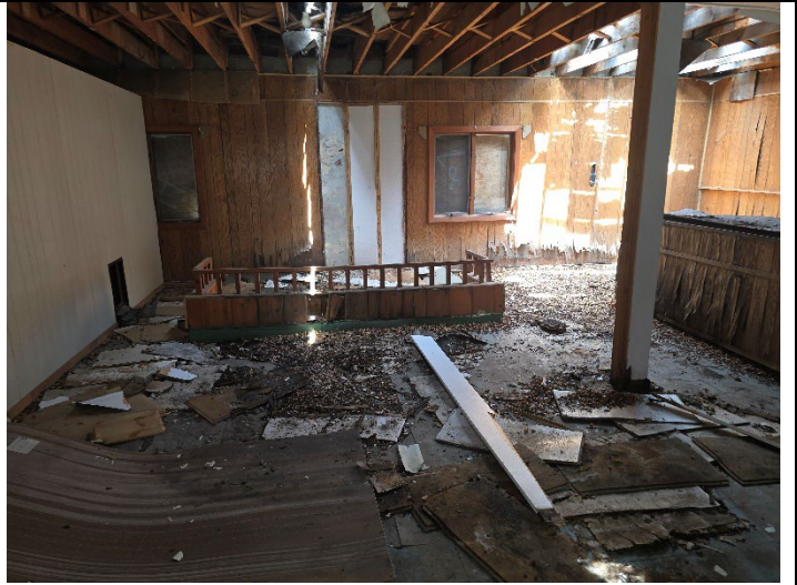
Photograph #2 –View of collapsed roof in the first floor office space. Extensive water damage was observed. Mold growth was present throughout the area. Flooring materials in this area are ACM.
