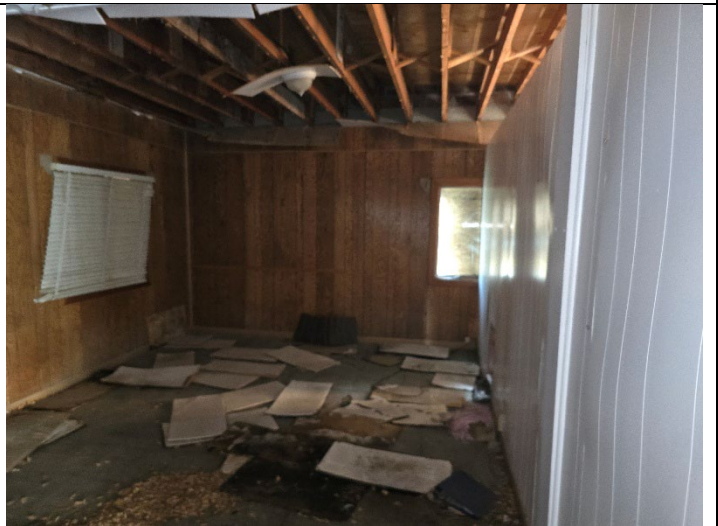
Photograph #4 – View of water damaged, mold impacted ceiling materials in the west office area. Flooring materials in this area are ACM.
