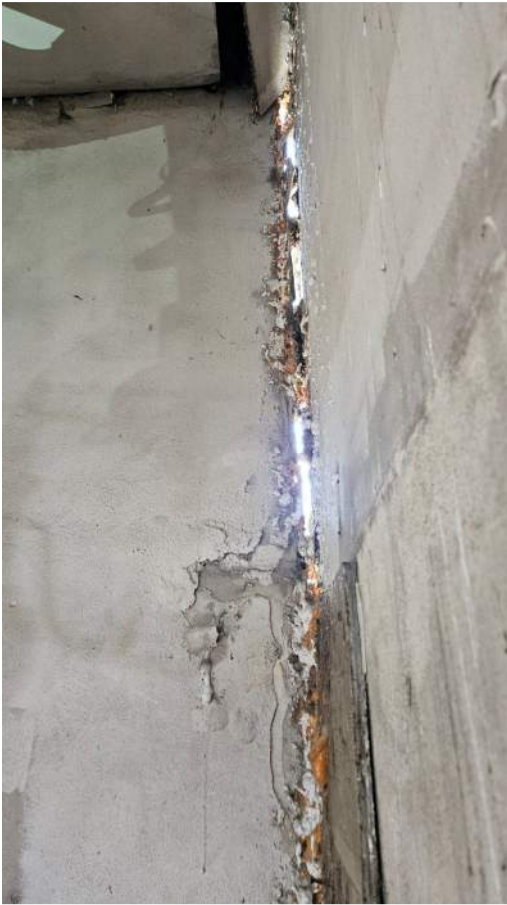
Figure B7 - Item S3 – Wall Crack in Shop portion of building.
