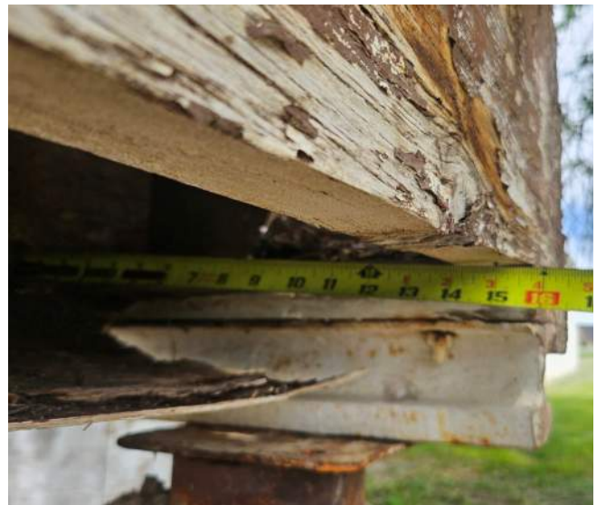
Figure A14 -Item S1, S2 – Office Wing Entry Foyer Floor Framing support beam- column condition – lack of positive connection.
