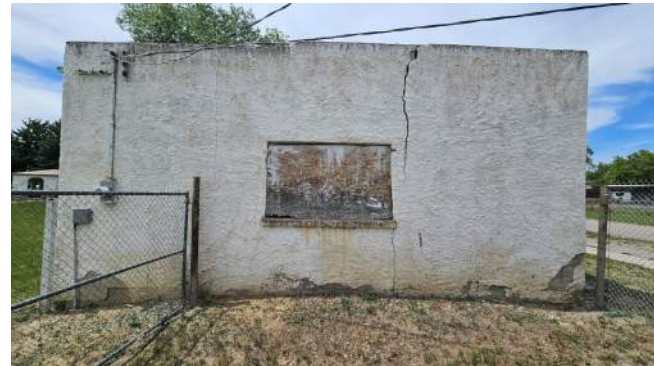
Figure B4 - Item S3 – East elevation of Shop portion of building – significant cracking exhibited.
