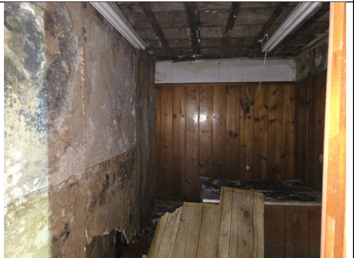
Photograph #8 – View of office area in the NE corner of the basement. Extensive water damage, mold growth and accumulation of pigeon guano was observed.
