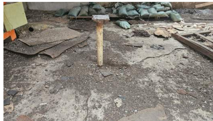
Figure B6 - Item S2 – Typical slab crack in Shop portion of building – significant cracking exhibited.
