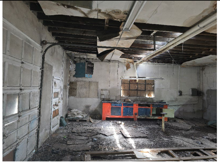
Photograph #10 – View of east end of the garage. The area has extensive water damage, mold growth, and heavy pigeon guano accumulation.
