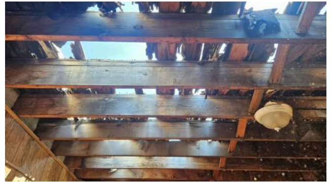
Figure A18 - Item S4 – Office wing partial roof decking collapse.
