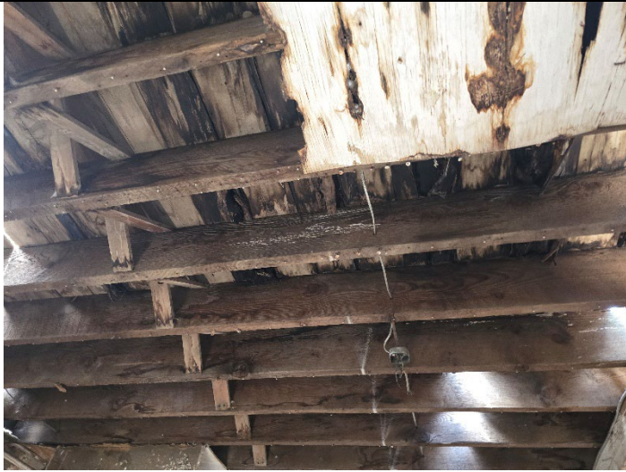
Photograph #9 – View of water damaged roof deck and ceiling materials in the garage area. Roof deck and roof joists are rotted.
