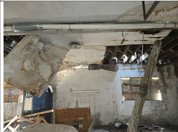
Photograph #3 –View of collapsed ceiling and roof in the garage area. Mold growth and pigeon guano are present throughout the area.
