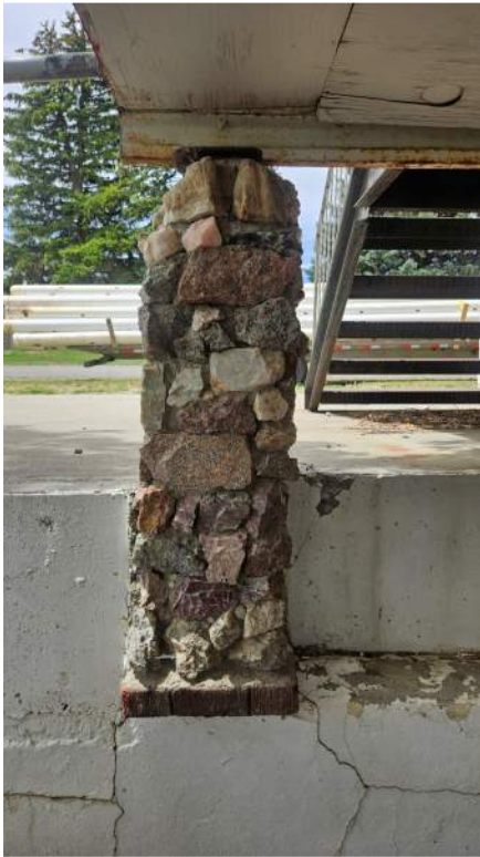
Figure A11 - Item S1, S2 – Office Wing Entry Foyer Floor Framing support column on severely cracked foundation wall.
