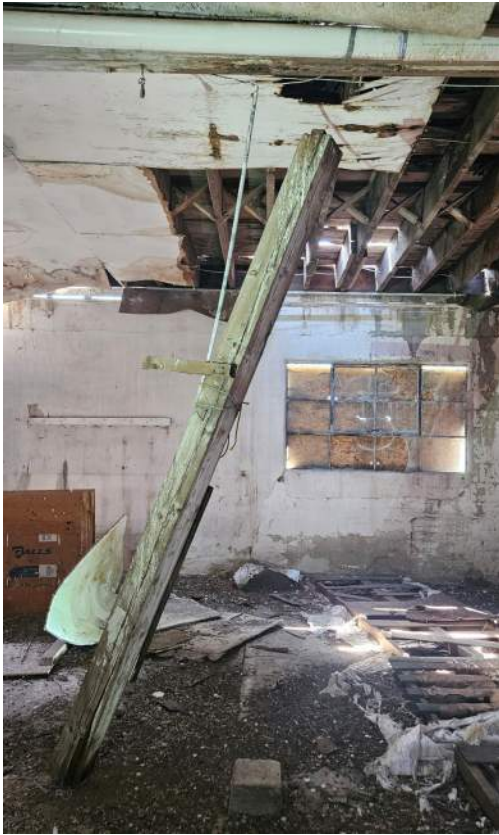
Figure B9 - Item S4 – Shop Wing failed roof beam support post.
