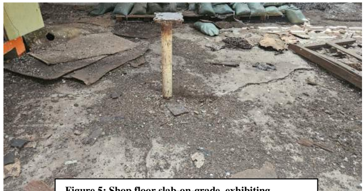
Figure 5: Shop floor slab-on-grade, exhibiting significant cracking and differential settlement.
