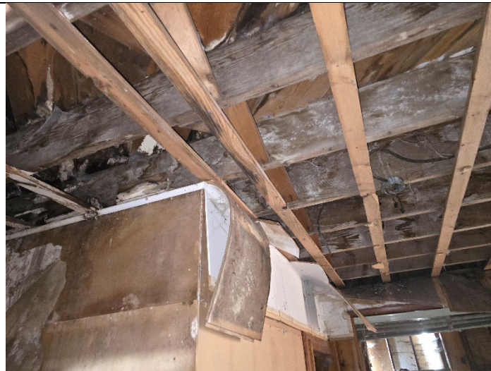
Photograph #7 – View of water damaged, rotted floor deck and floor joists above basement area.
