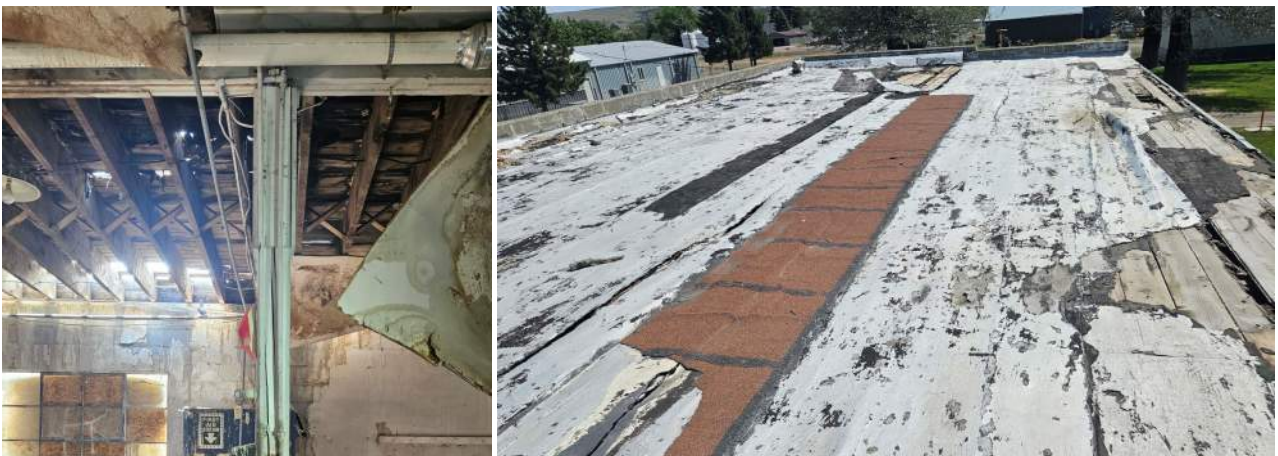
Figure 10a: (Left) View of built-up beam supporting Shop rafters, with deterioration and decay present throughout, and partial decking collapse allowing exposure to the elements; 10b (Right) View of exterior roof surface of the Shop Wing, looking to the east; partial roof decking collapse/failure throughout.
