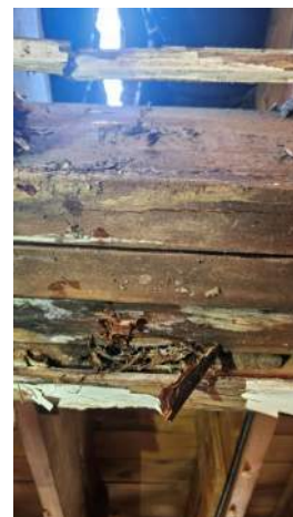
Figure A2 – Item S4 – Close up view of beam deterioration over Office Wing.
