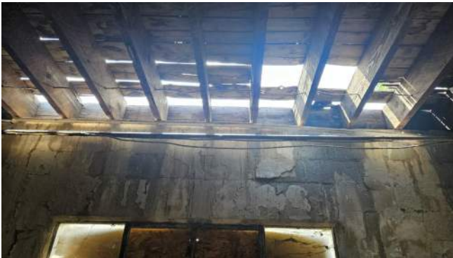
Figure B11 - Item S4 – Shop wing partial roof decking collapse.
