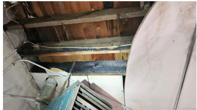
Figure B12 - Figure B12 - Item S4 – Shop Wing charred roof rafters.
