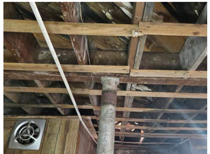
Figure A10 - Item S2 – Office wing floor framing, wood joists attached to steel beam with no positive connection.
