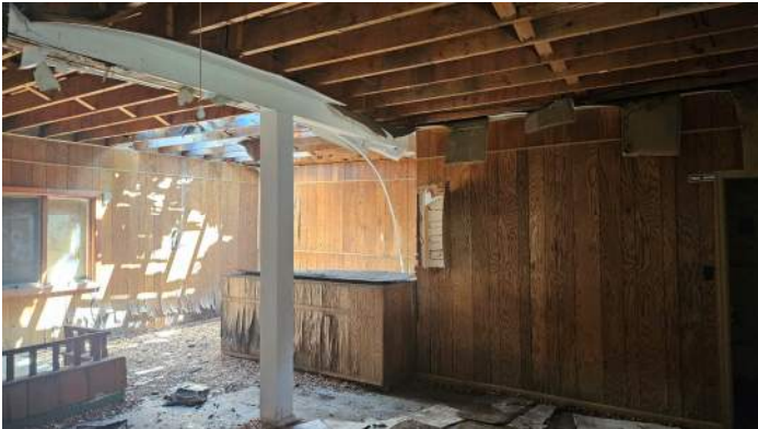
Figure A17 - Item S4 – Typical Roof Framing over Office Wing – partial roof decking collapse.
