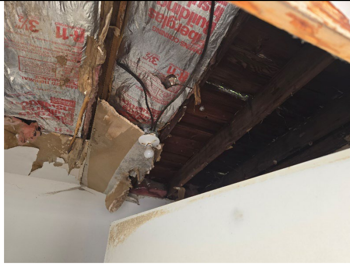
Photograph #5 –View of rotted roof deck and roof joists.
