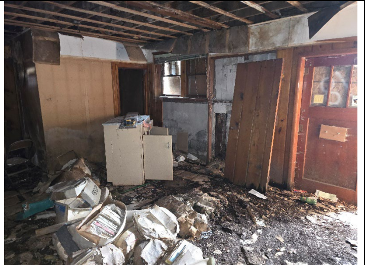
Photograph #6 – View of basement area. Extensive water damage, mold growth and accumulation of pigeon guano was observed. Flooring materials in this area are ACM. Records are water damaged, moldy and covered with pigeon guano.
