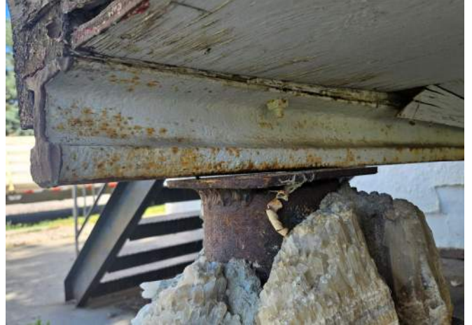
Figure A12 - Item S1, S2 – Office Wing Entry Foyer Floor Framing support beam- column condition – lack of positive connection.
